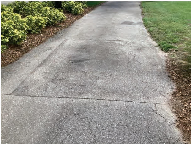
Cracks and previous repairs evident
