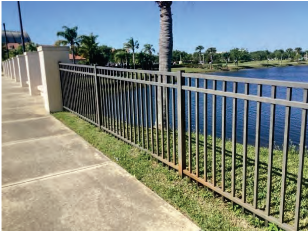
Railings – finish fade evident
