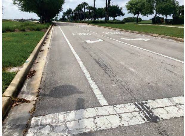
Pope John Paul II Blvd. – deterioration evident
