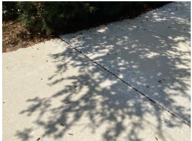
Concrete sidewalks – grinding repairs evident
