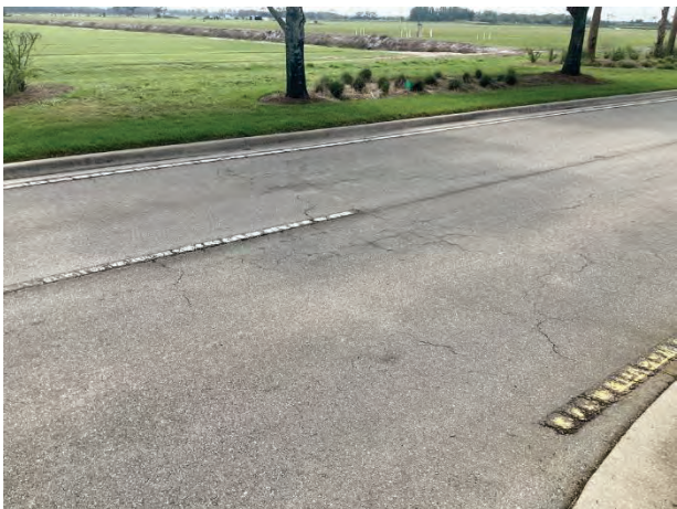
Ave Maria Blvd. – cracks evident
