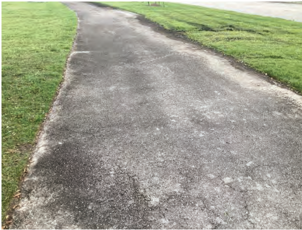
Deterioration of the pavement evident
