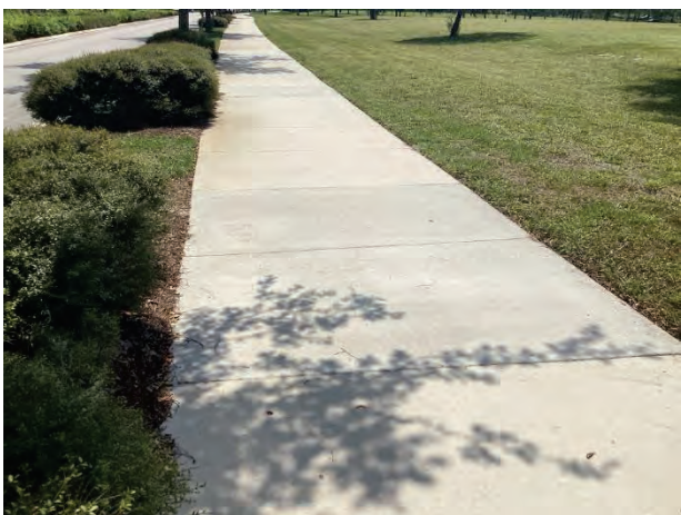
Concrete sidewalks – previous partial replacements evident
