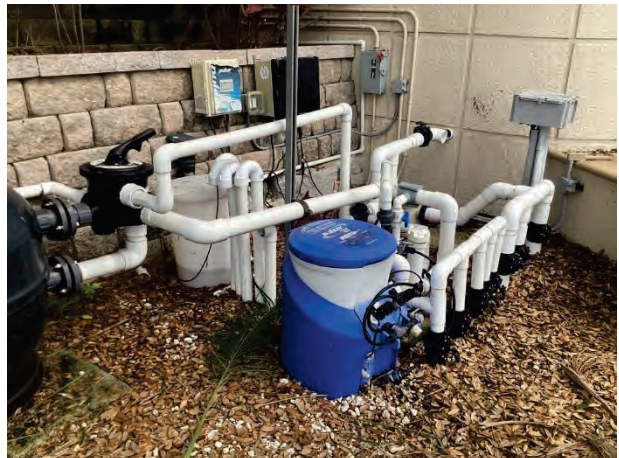
Typical mechanical equipment
