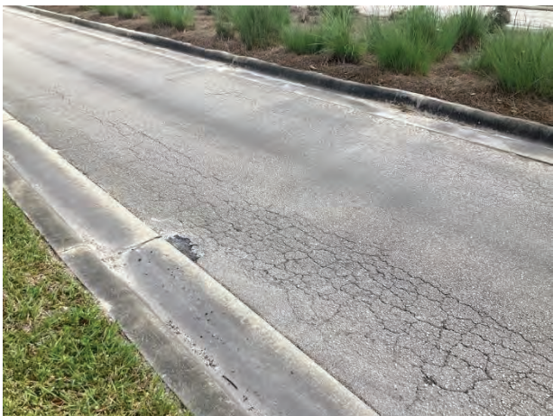
Pope John Paul II Blvd. – alligator cracking and raveling evident
