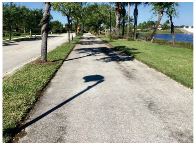
Asphalt pavement walking path at Lake Park – minor deterioration evident
