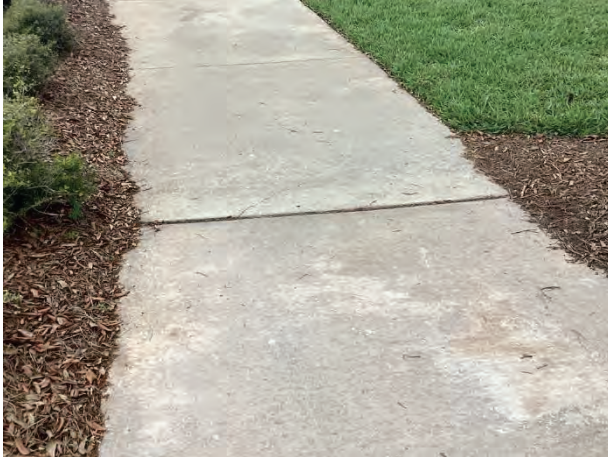
Concrete sidewalks – Pope John Paul II Blvd. – uplift evident
