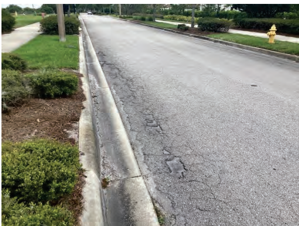
Pope John Paul II Blvd. – cracks and top layer deterioration evident
