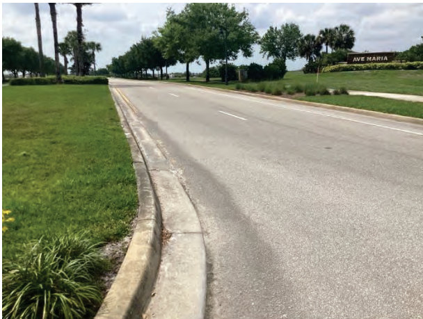
Pope John Paul II Blvd. – deterioration evident
