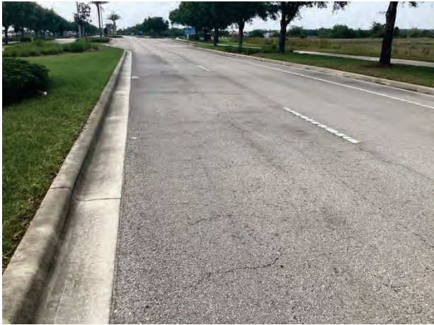
Pope John Paul II Blvd. – cracks and raveling evident
