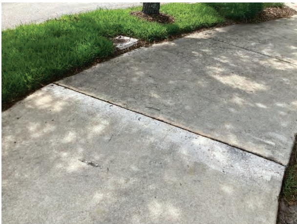
Concrete sidewalks – Pope John Paul II Blvd. – grinding repairs evident
