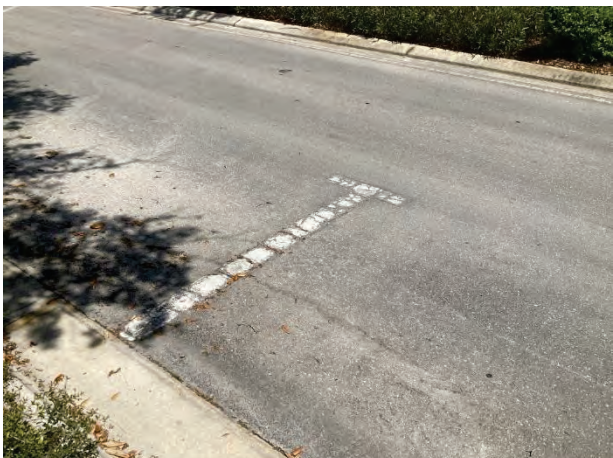
Ave Maria Blvd. - cracks and raveling evident
