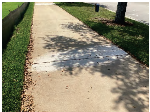
Concrete sidewalks – Anthem Parkway – grinding repairs evident
