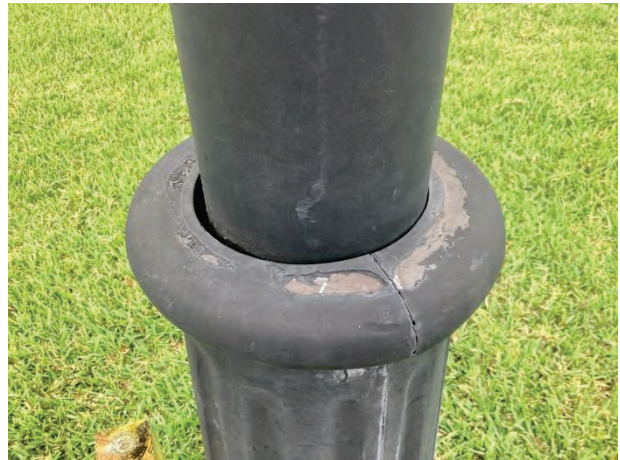
Light poles and fixtures – galvanized – finish fade evident
