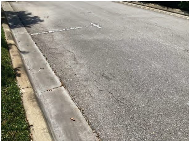
Ave Maria Blvd. - cracks and raveling evident
