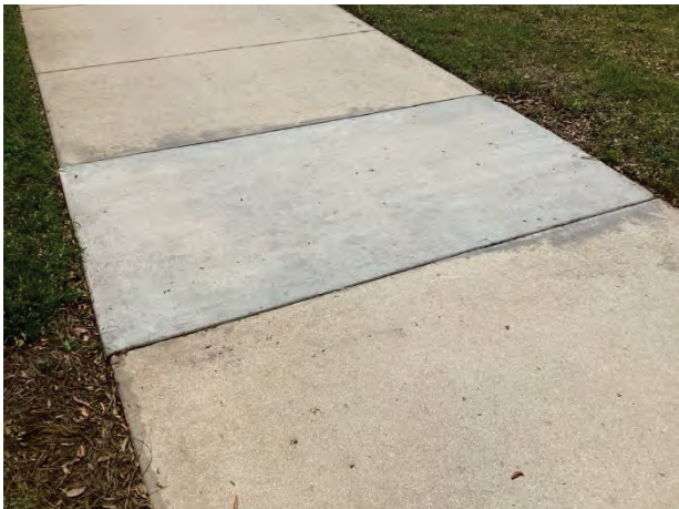
Concrete sidewalks – previous partial replacements evident
