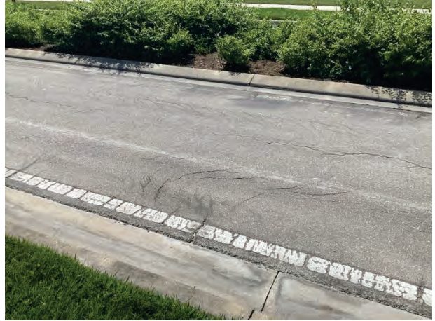
Ave Maria Blvd. – slippage cracks evident
