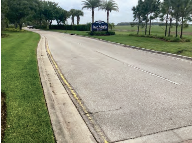
Ave Maria Blvd. – cracks evident
