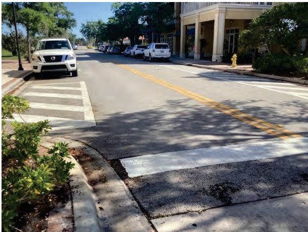
Seton St. – deterioration evident
