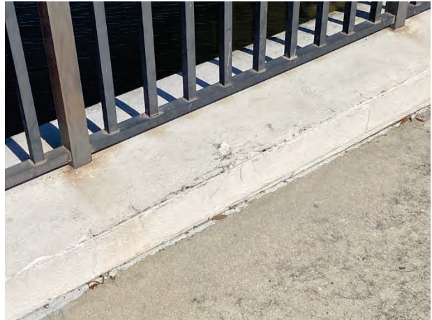
Coating fade evident
