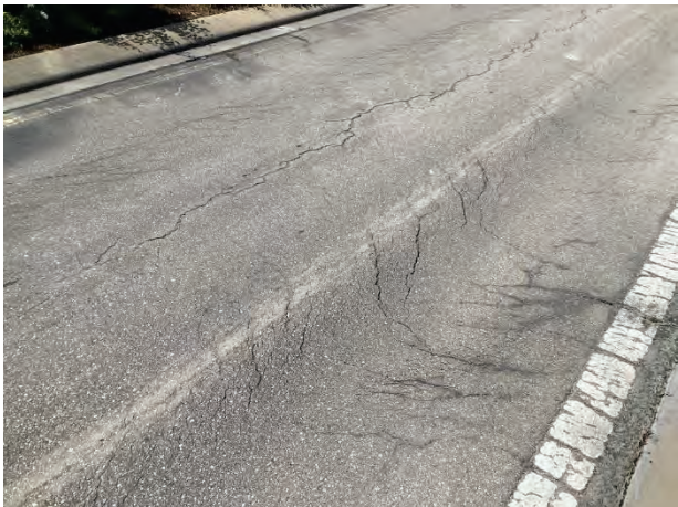
Ave Maria Blvd. – slippage cracks evident
