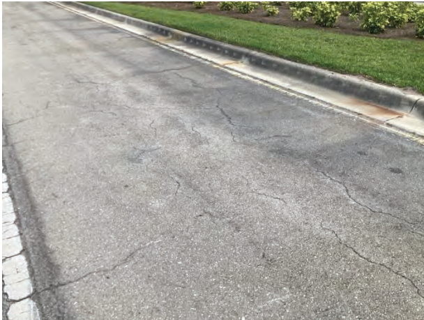
Ave Maria Blvd. – cracks and raveling evident
