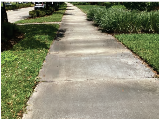
Concrete sidewalks - Ave Maria Blvd. – uplift evident
