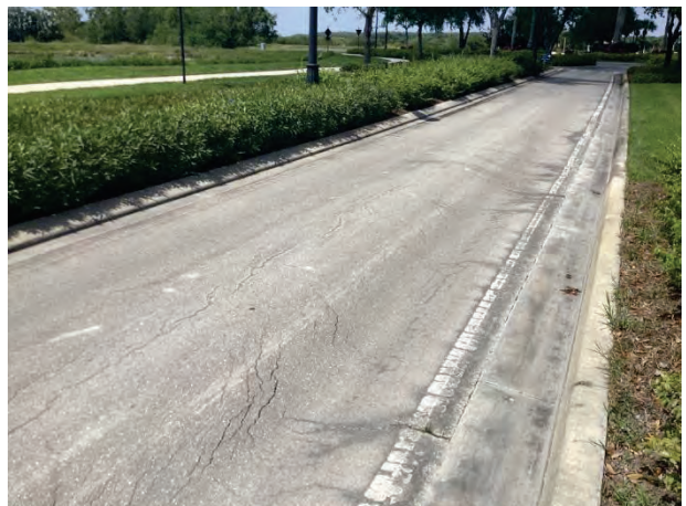
Ave Maria Blvd. - cracks and raveling evident
