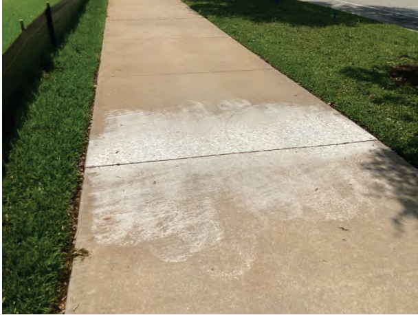
Concrete sidewalks – Anthem Parkway – grinding repairs evident
