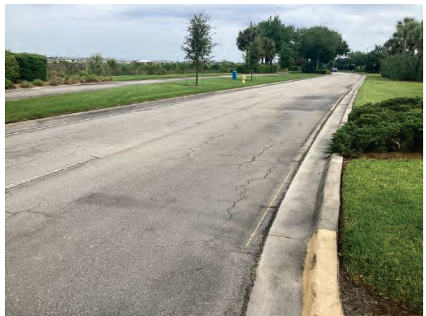
Ave Maria Blvd. – cracks and raveling evident
