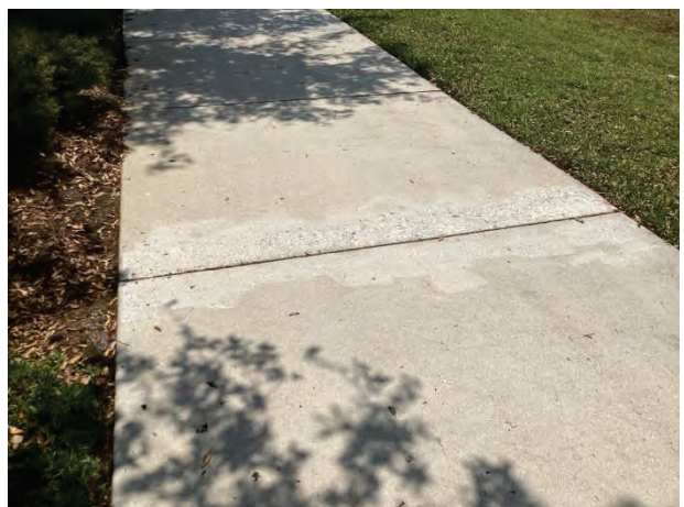
Concrete sidewalks – grinding repairs evident
