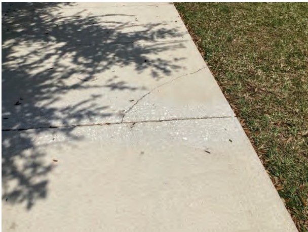
Concrete sidewalks – cracks and grinding repairs evident
