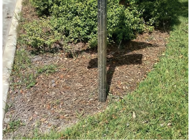
Signage – finish fade evident
