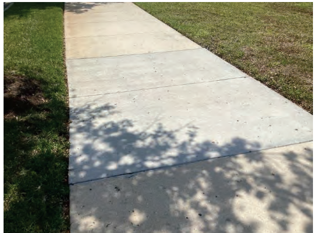
Concrete sidewalks – previous partial replacements evident
