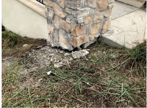
Oil Well Rd. entrance – damaged masonry evident
