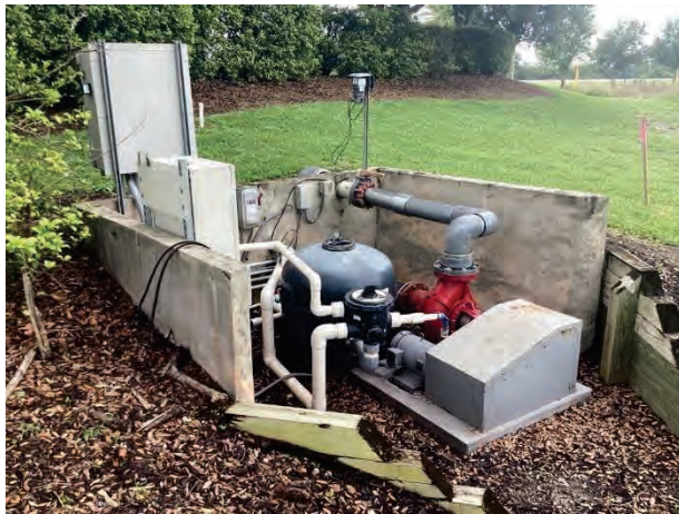
OWR mechanical equipment - overview
