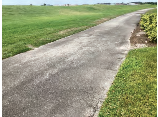
Deterioration of the pavement evident
