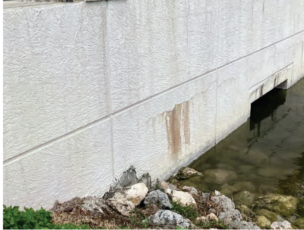
Pope John Paul II Blvd. – coating deterioration evident
