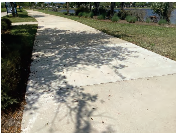
Concrete sidewalks – grinding repairs evident
