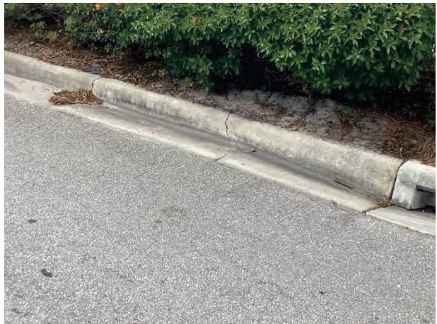
Concrete curbs and gutters – minor cracks evident
