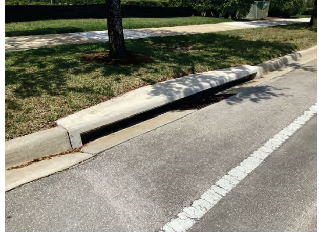
Catch basin - typical
