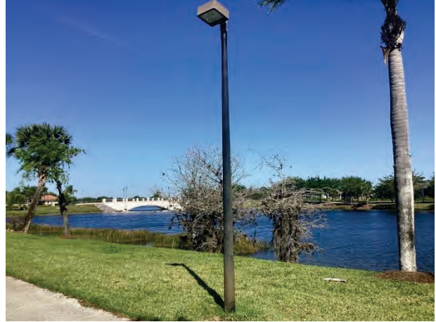
Light poles and fixtures – fiber glass – finish fade evident
