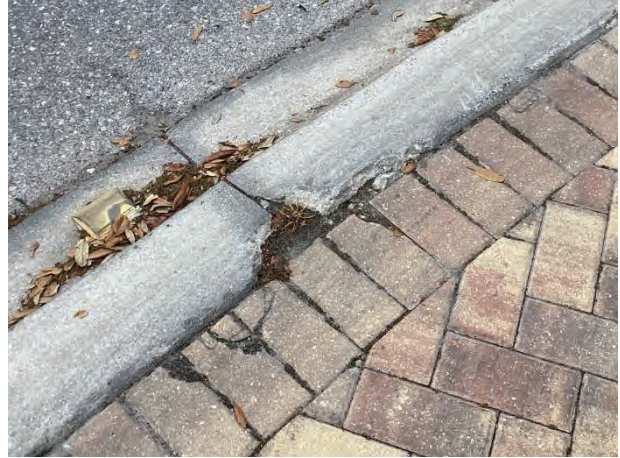
Concrete curbs and gutters – deterioration of the concrete evident
