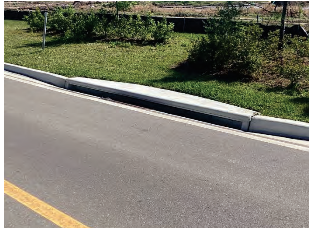
Catch basin - typical
