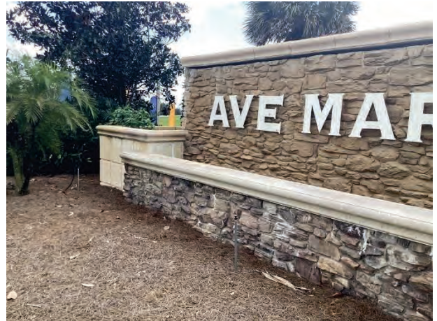
CKR Stone veneer - minor efflorescence evident
