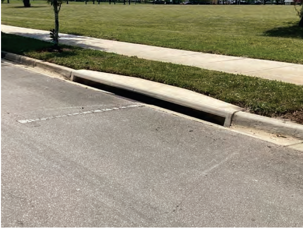
Catch basin - typical
