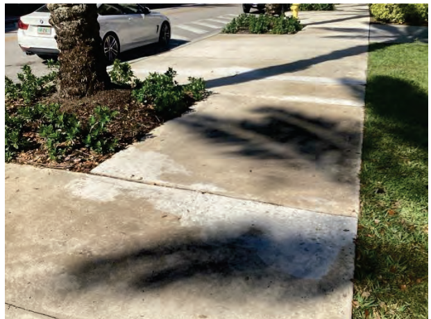
Concrete sidewalks – grinding repairs evident
