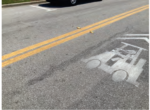
Ave Maria Blvd - deterioration evident
