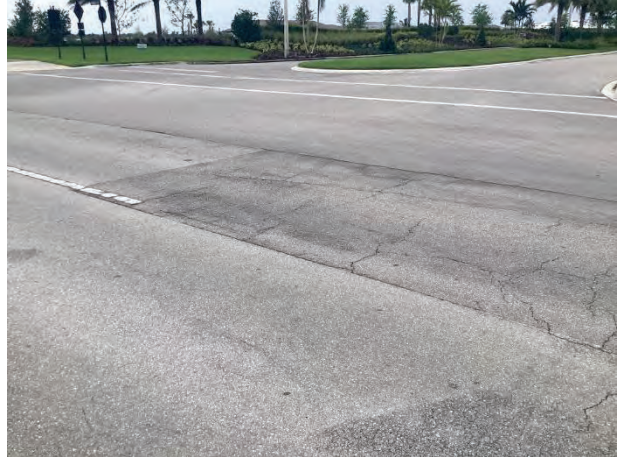
Ave Maria Blvd. – cracks and raveling evident
