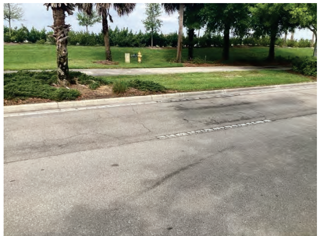
Ave Maria Blvd. – cracks and raveling evident
