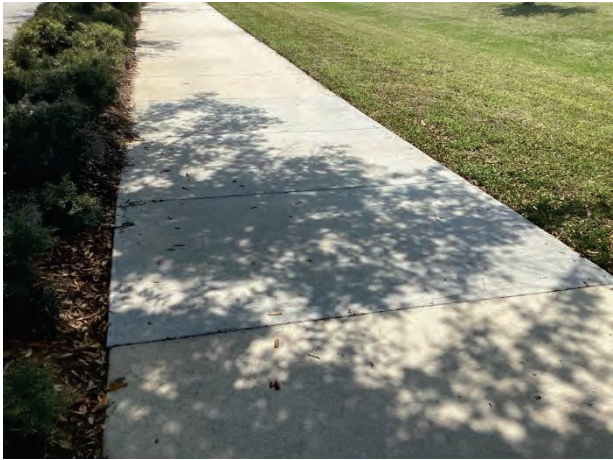
Concrete sidewalks – grinding repairs evident
