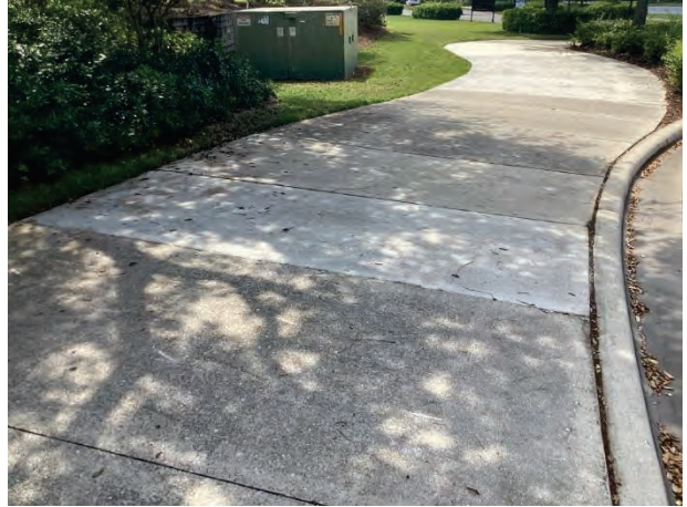
Concrete sidewalks - Ave Maria Blvd. – previous patch repairs evident
