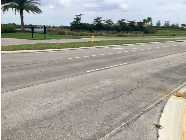
Ave Maria Blvd. – cracks and raveling evident
