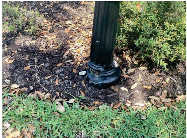
Signage – damage evident
