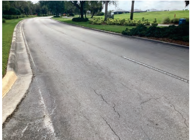
Ave Maria Blvd. – cracks and raveling evident
