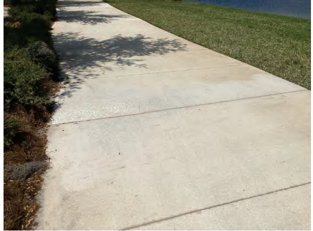
Concrete sidewalks – grinding repairs evident
