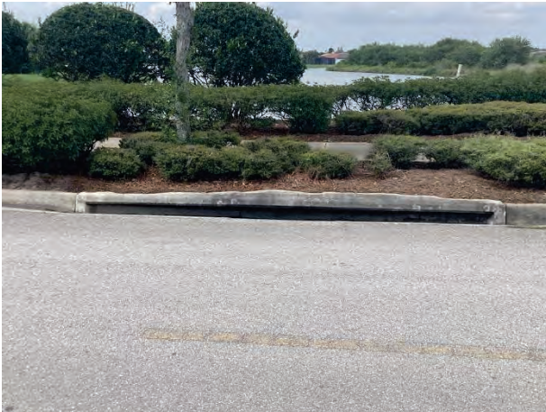
Catch basin - typical
