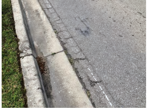
Ave Maria Blvd. – deterioration of the striping evident
