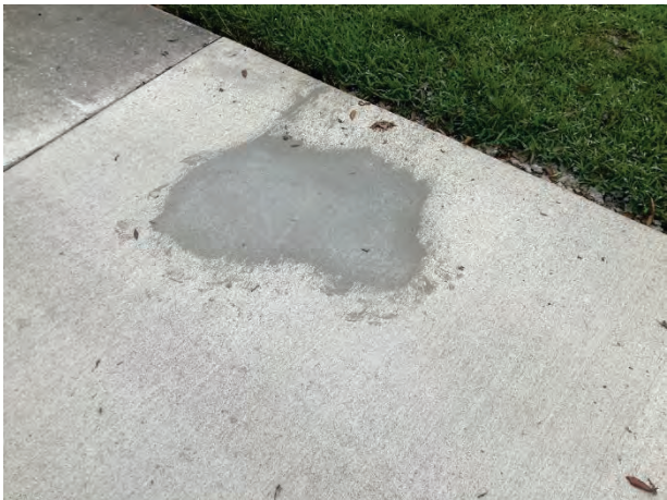
Concrete sidewalks – patch repairs evident
