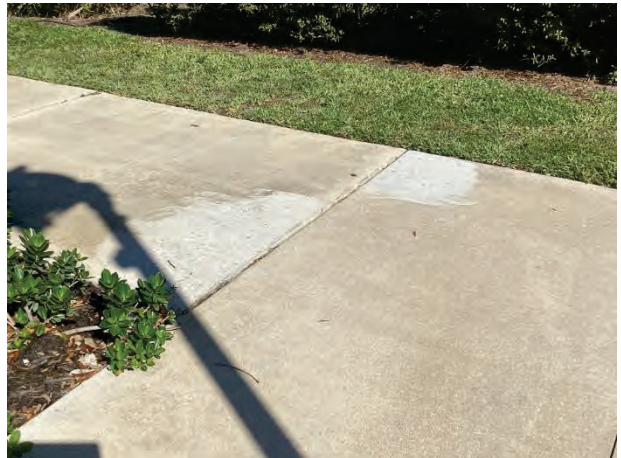
Concrete sidewalks – grinding repairs evident
