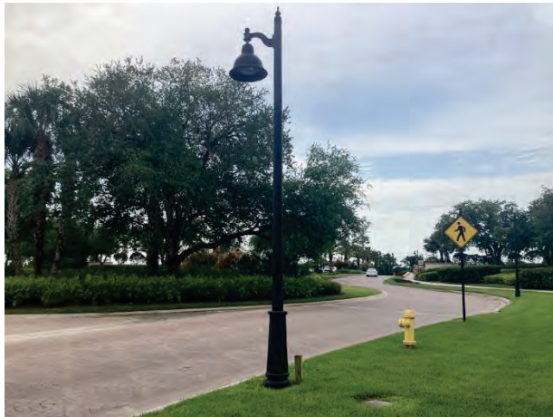
Light poles and fixtures – galvanized - overview
