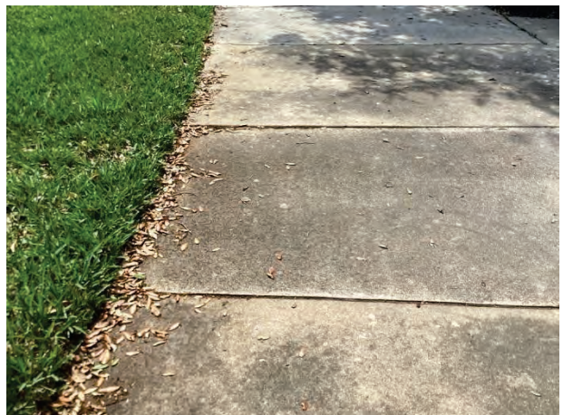
Concrete sidewalks - Ave Maria Blvd. – uplift evident
