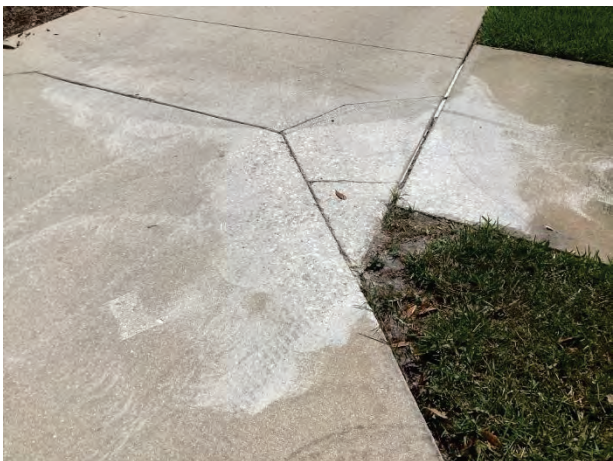
Concrete sidewalks - Ave Maria Blvd. – gridding repairs evident
