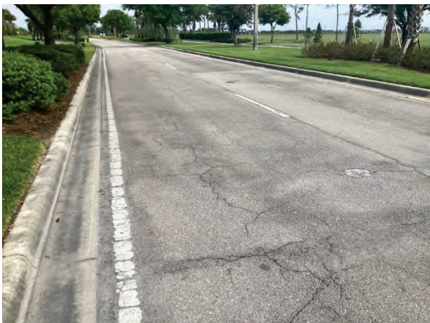
Ave Maria Blvd. – cracks and raveling evident
