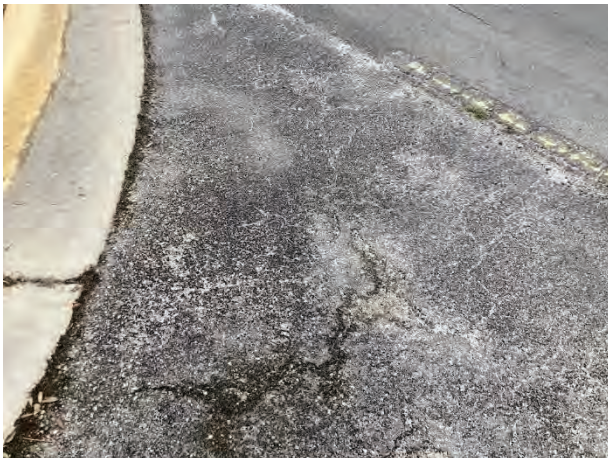
Ave Maria Blvd – deterioration evident
