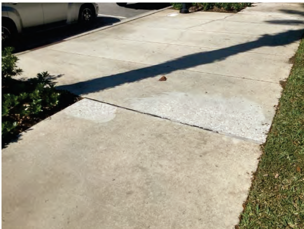
Concrete sidewalks – grinding repairs evident
