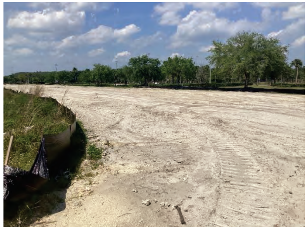
This is asphalt pavement that was under construction during our inspection. Future updates to this Reserve Study should consider additional quantities and conditions.
